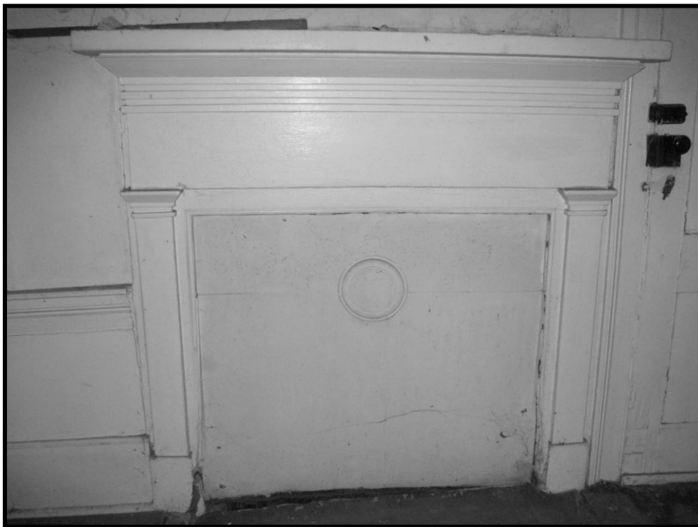
Figure 68 No. 126 Love House, Interior, First Floor, Detail of Mantel on Southeast Gable End.
