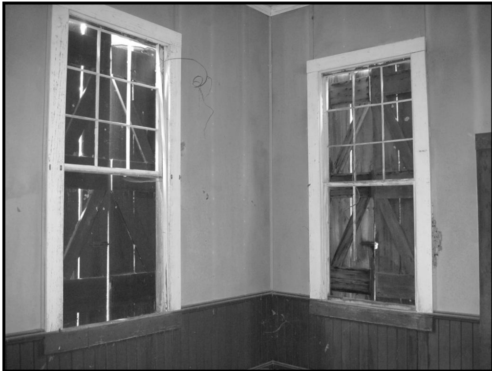
Figure 76. No. 135 Former Weyman Methodist Church, Interior, View of Original Sash Windows, Looking South.
