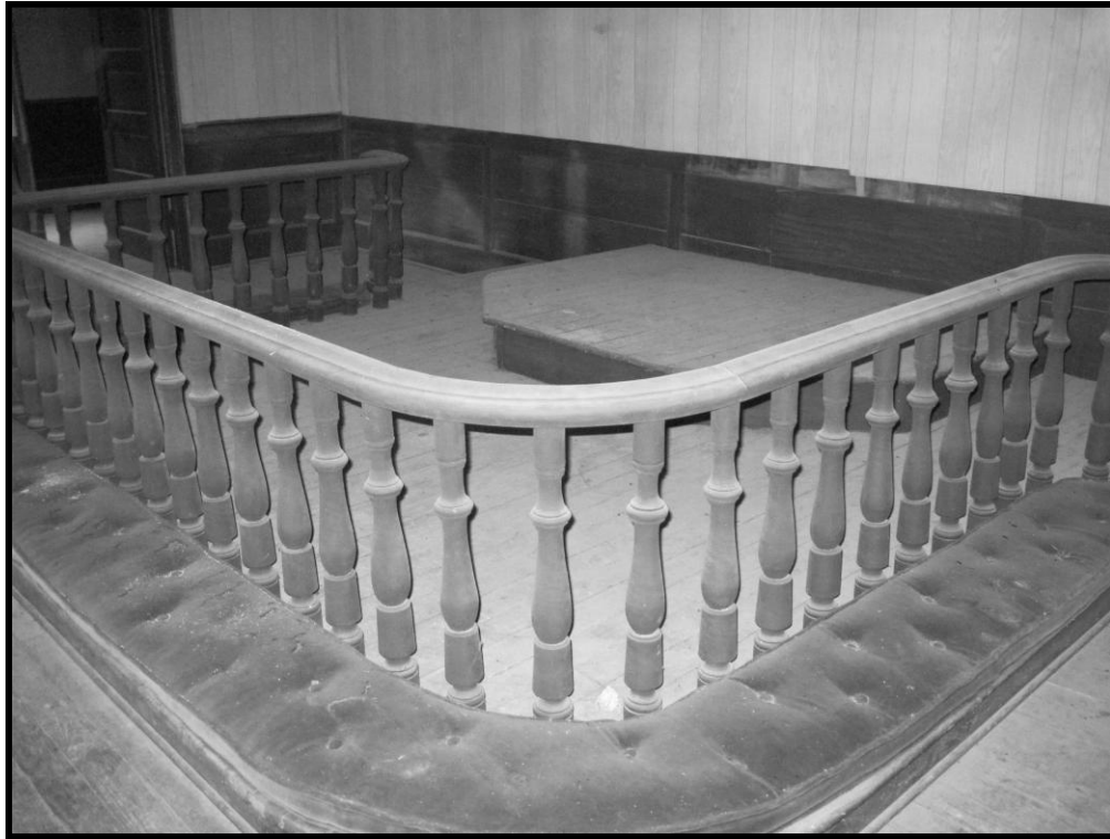
Figure 81. No. 135 Former Weyman Methodist Church, Interior, Detail of Altar Rail, Looking North.
