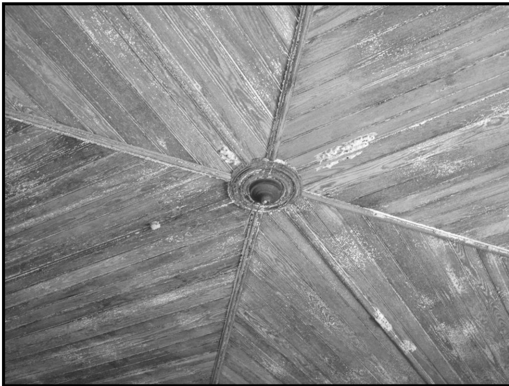
Figure 80. No. 135 Former Weyman Methodist Church, Interior, Detail of Ceiling and Remnant of Light Fixture.
