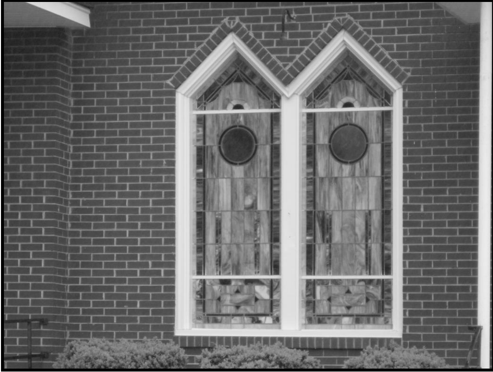
Figure 47. No. 76 Carvers Creek AME Zion Church and Cemetery, Detail of Window on West Elevation.
