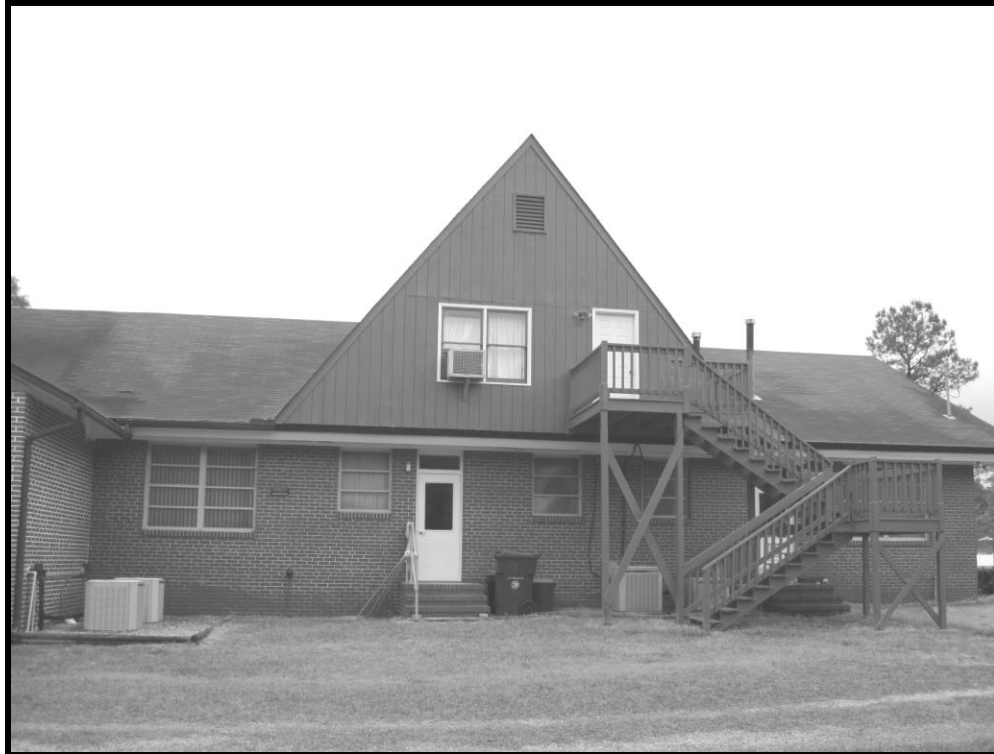
Figure 112. No. 169 Wesley United Methodist Church, View of Northeast Elevation Showing 1987 Addition, Looking Southwest.
