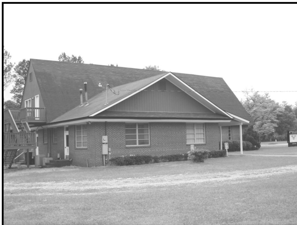
Figure 113. No. 169 Wesley United Methodist Church, View of Northwest Elevation of Original Wing, Looking South.
