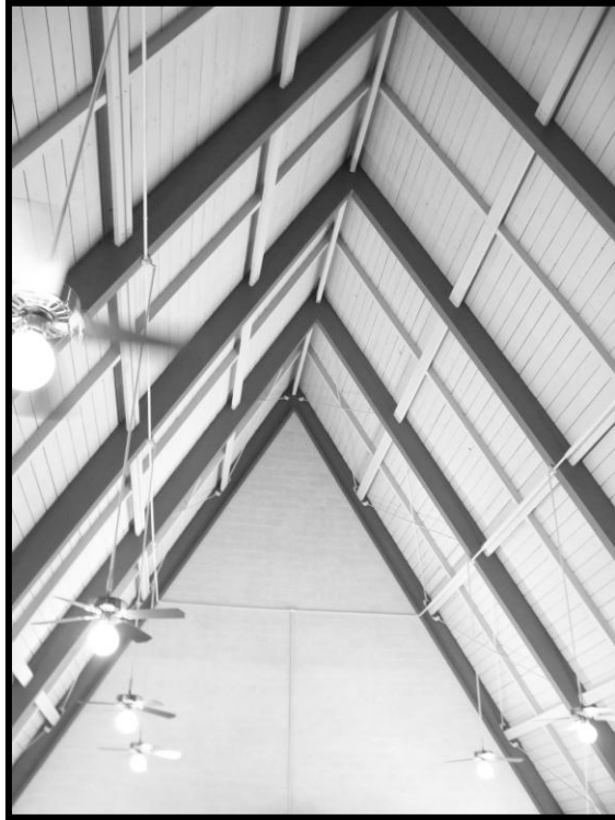
Figure 102. No. 163 Acme Presbyterian Church, Interior, View of Ceiling in Sanctuary, Looking Northeast.
