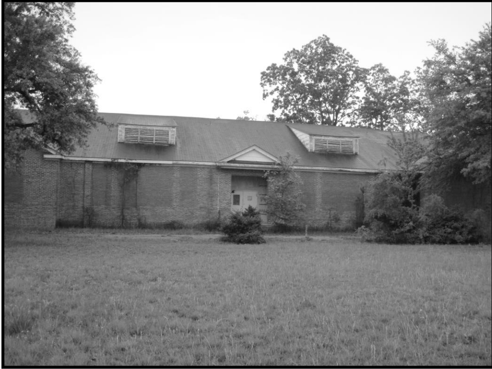
Figure 52. No. 77 Carvers Creek School, View of Northeast Elevation of School, Looking Southwest.
